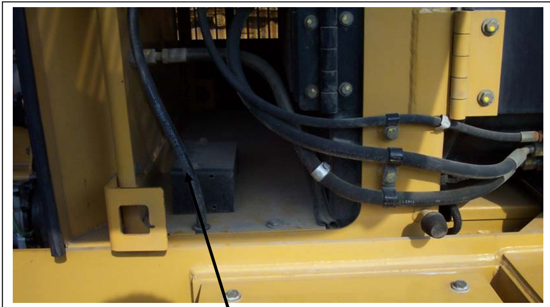
5/16" line running out of the radiator compartment and up towards the cab.
